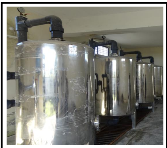
Water Tanks & Filtration Unit Cost 54.44 M
